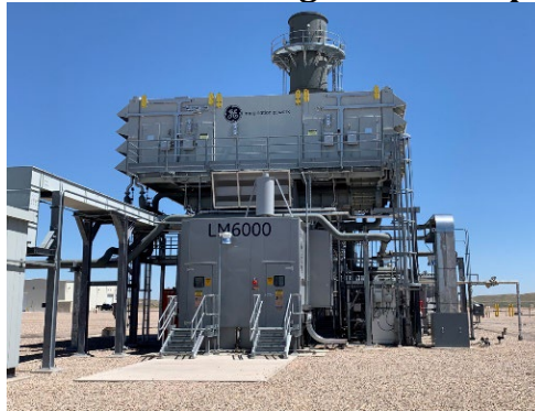
Figure 05-3 Cheyenne Prairie Generating Station Simple Cycle CT
